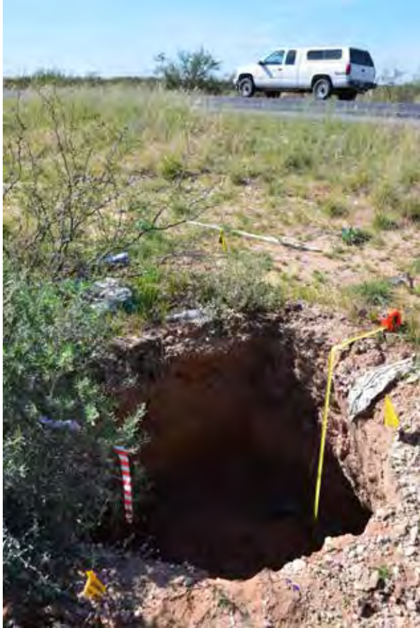
Figure A10. Station 9.7 sinkhole in road base.
