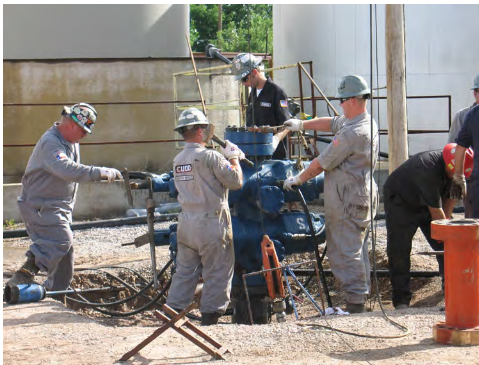
Figure 13. Workers from CUDD Energy Services locking down a blowout preventer on Eugenie #1 on 10 July 2010 to prevent additional flow of brine. Photo by George Veni.
